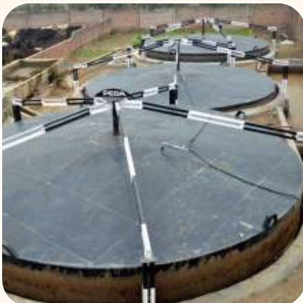
Waste to Energy
